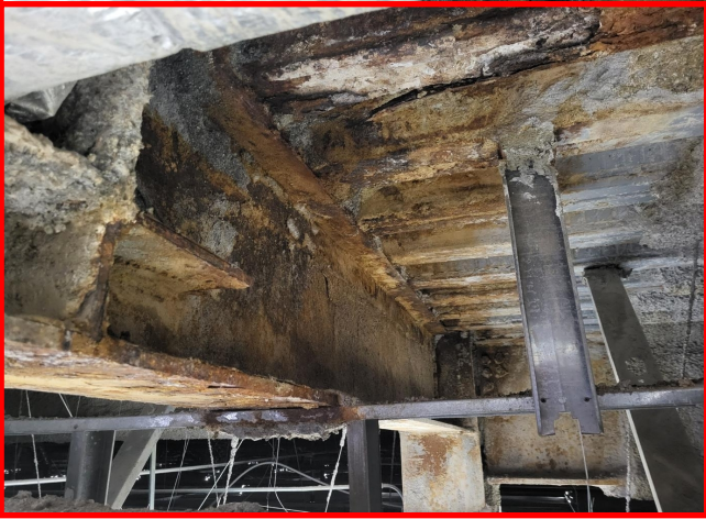
Rusted beams, deck and hangers
