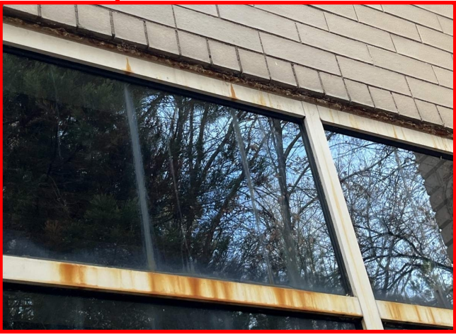
Rusted ledgers and window system at basement wall
