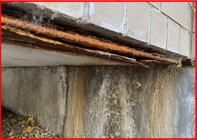
Rusted ledgers and cracked brick veneer at bridge
